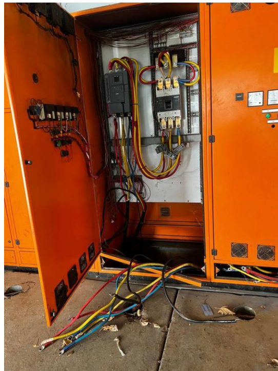
Pump 2 Electric box condition open
