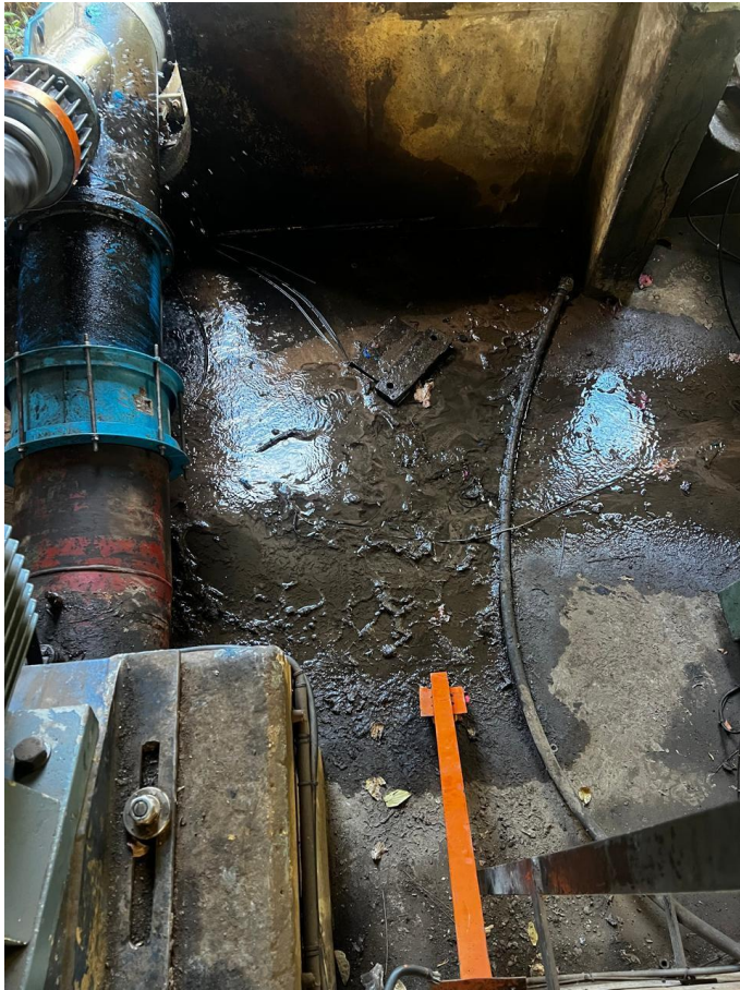
Water leaking from pump 1 at a rapid speed. Picture taken 5 June 2026.
