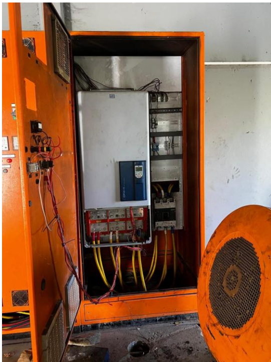
Pump 1 Electric box condition open
