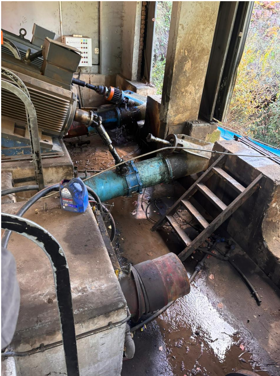
Raw water pump station: Pump 1 – Aging pump, leaking water. Pump 2 – Disconnected. Pump 3 – No pump and pipes are removed. Picture taken 5 June 2026.
